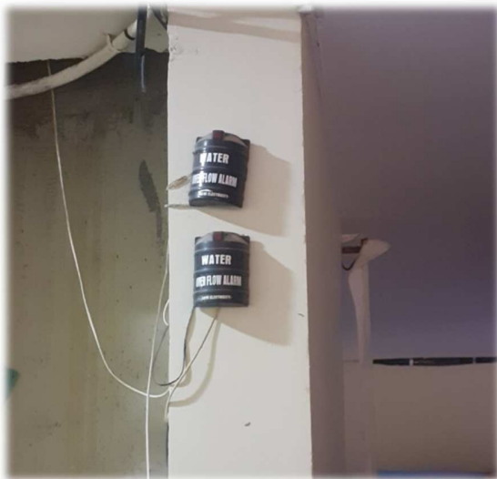
Water sensors to avoid water wastage
