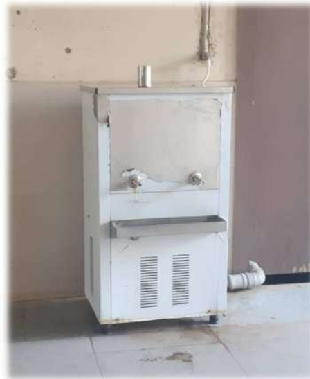
Drinking water filters and coolers
