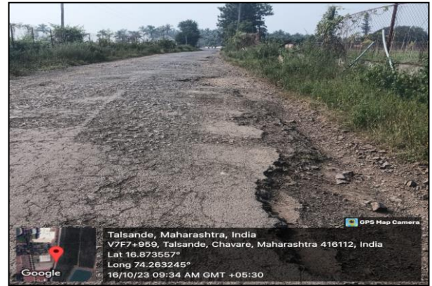
Defected Edge of Road
